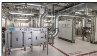
Gambar 2.38. Filter udara BSL 3
